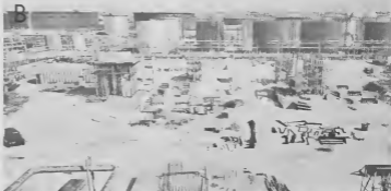
Site of hydrogen units, looking north from Powerhouse No. 1. Sitio di unidadnan hidrogeno, mirando noord for di Powerhouse No. 1.
